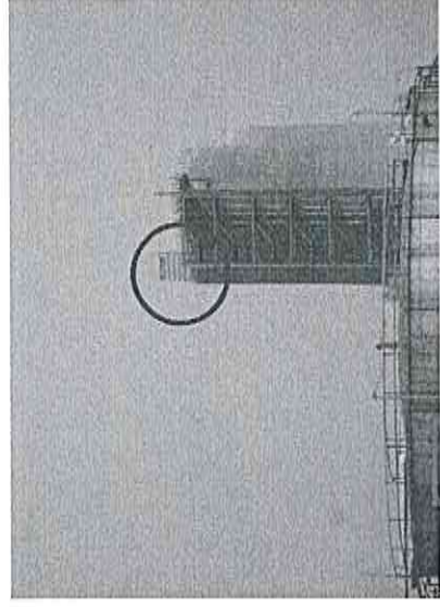
Bag Filter installed at Ash silo
